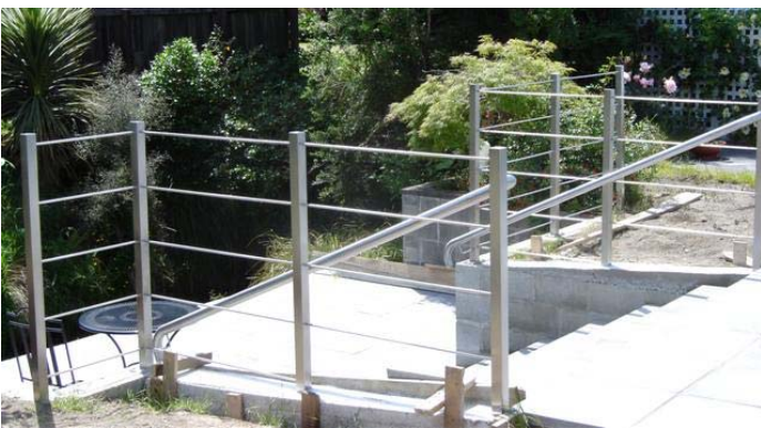
Stainless Steel Horizontal Fence and Handrails
